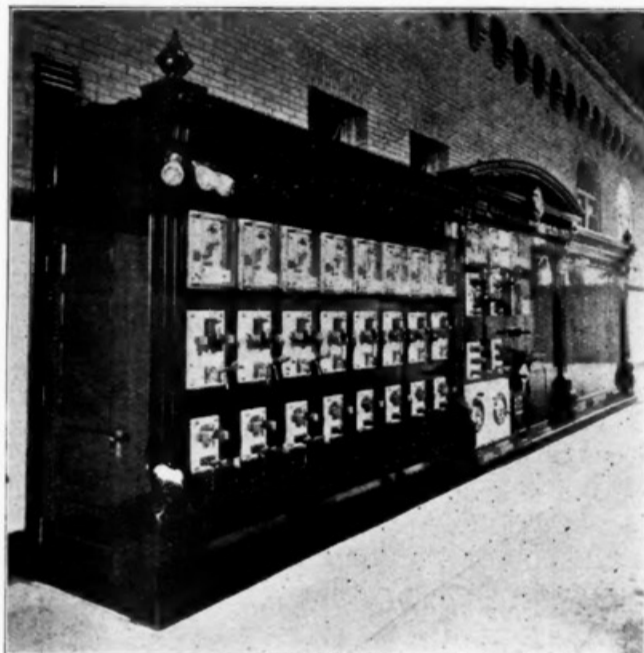
FIG. 3.—SWITCHBOARD IN COLUMBUS CENTRAL RAILWAY COMPANY'S POWER STATION.
